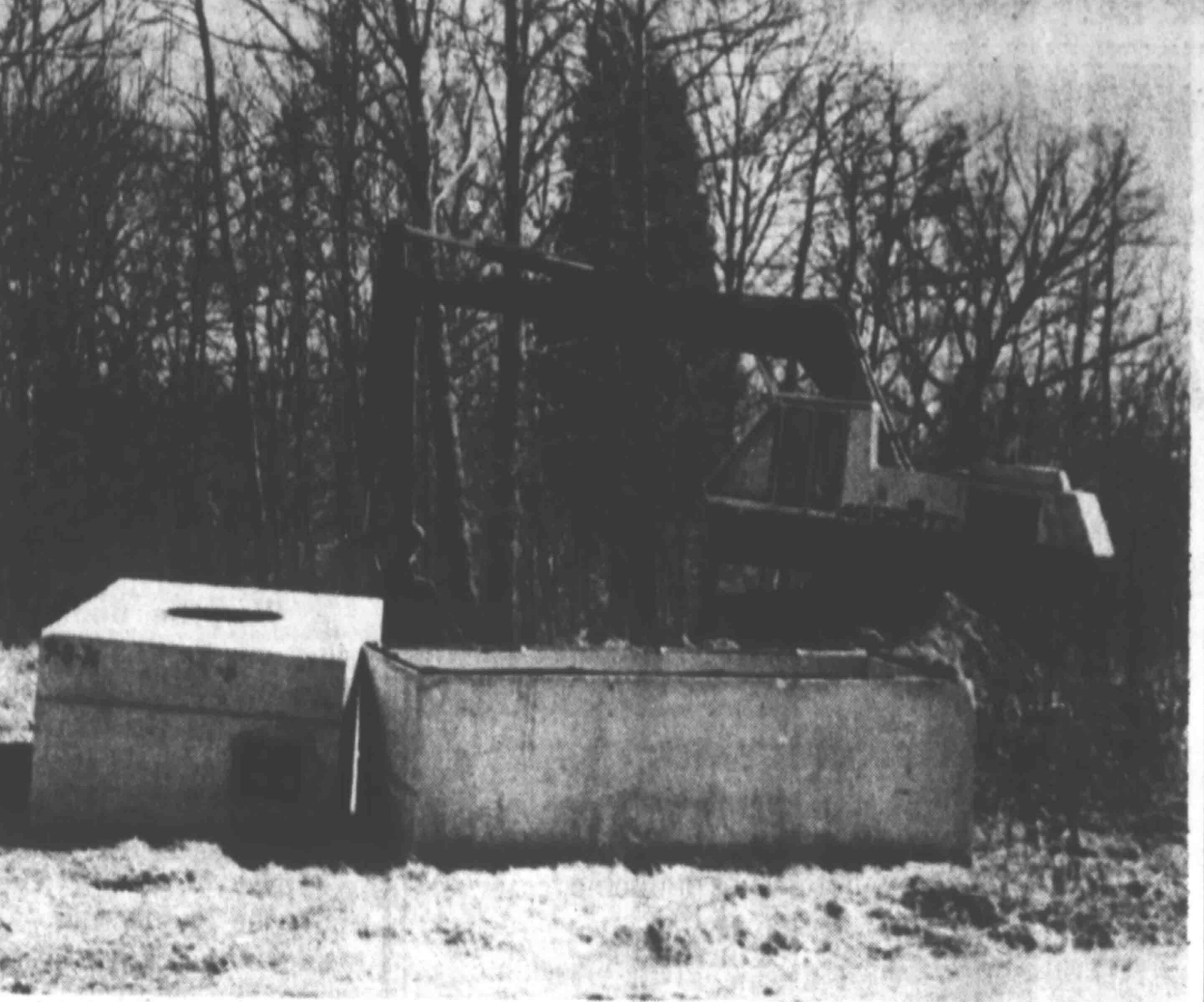
20 TELEPHONE MANHOLES ARE BEING INSTALLED between Ripley and Dyersburg by South Central Bell. The manholes provide seven feet of head space for men working on underground cables.
